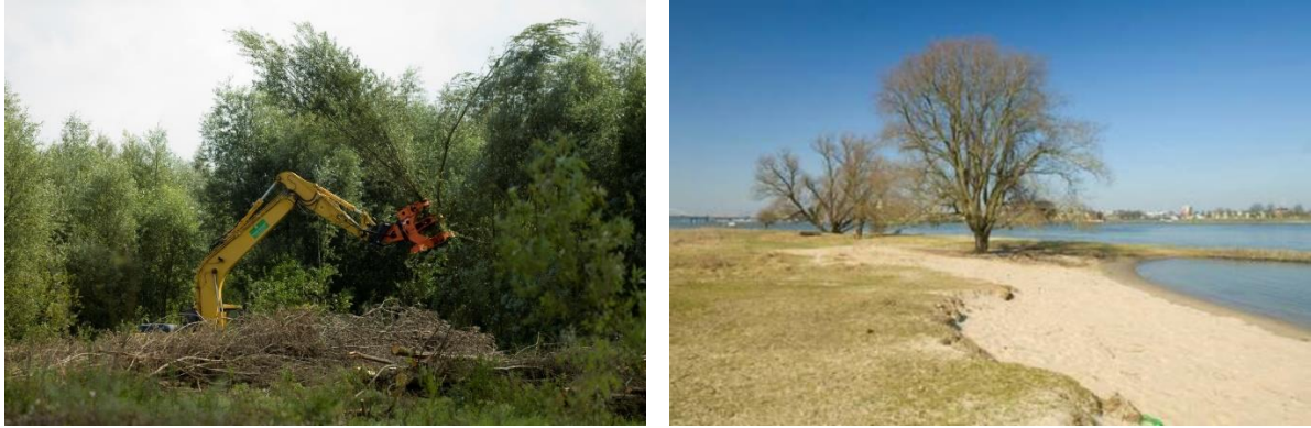
Figure 15 Managing vegetation in the Room for the River Project (removing trees to create more space for the river (left) and after a regular maintenance (right), source: Room for the River).
