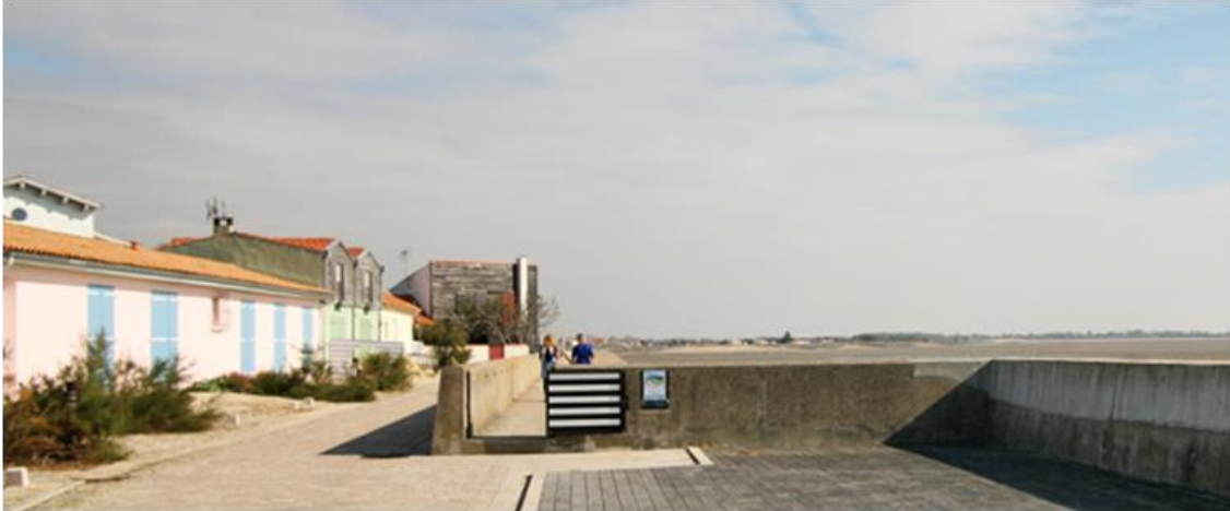
Figure 10-5 Reinforcement of the protection wall in les Boucholeurs with cofferdams along the walk path
