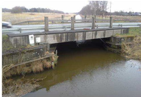
Figure 7-2 Measuring station in the outlet of Egå Engsø
