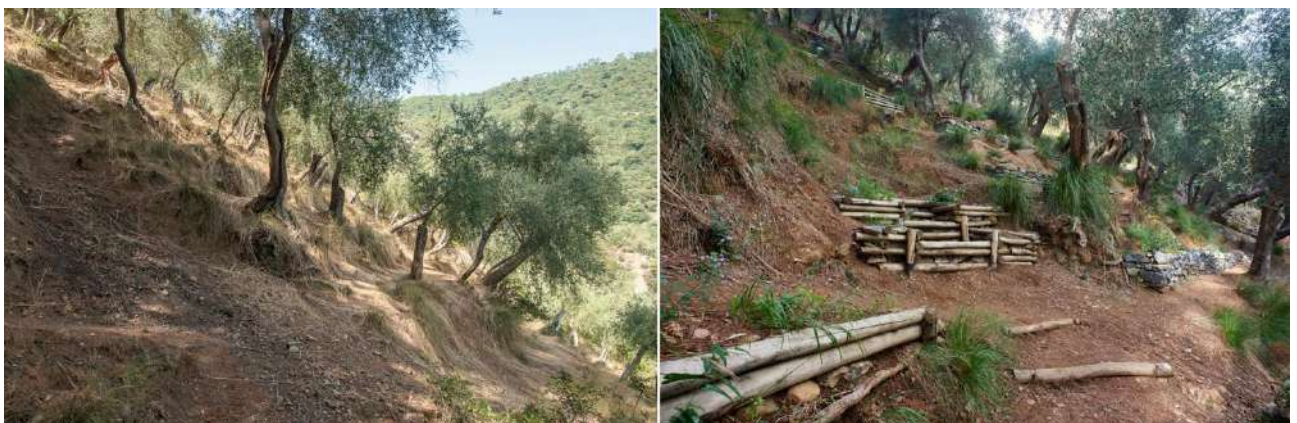
Figure 38 Terraces recovery in the San Fruttuoso historical olive orchard: the comparison between the before condition, on the left, and final one, on the right. Terraces have been recovered reconstructing the stone walls, while bioengineering
