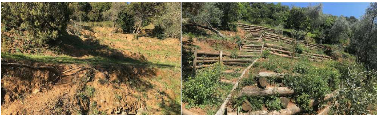
Figure 40 Terraces recovery in the Paraggi catchment - area 2: comparison between the before condition, on the left, and final one, on the right. The use of the less expensive bioengineering techniques than stone walls is compatible with the superintendence rules.
