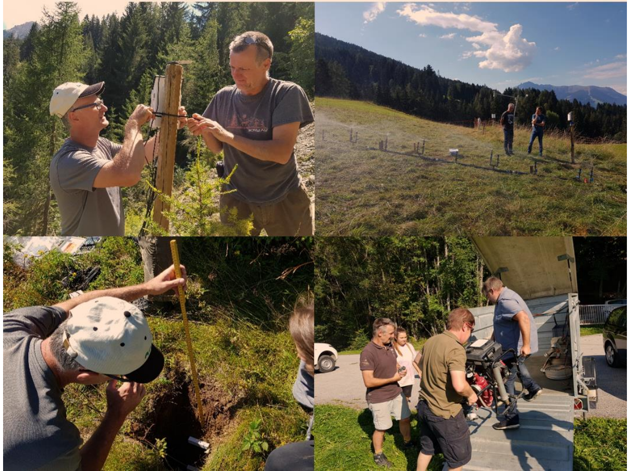
Figure 6: Installation of equipment in the field together with subcontractor BFW (Austrian Research Centre for Forests). The left two pictures are made of the installation of soil moisture sensors on August 5, 2020. The right two pictures are taken at the artificial rainfall-runoff site during a National Workshop on September 16, 2020.
