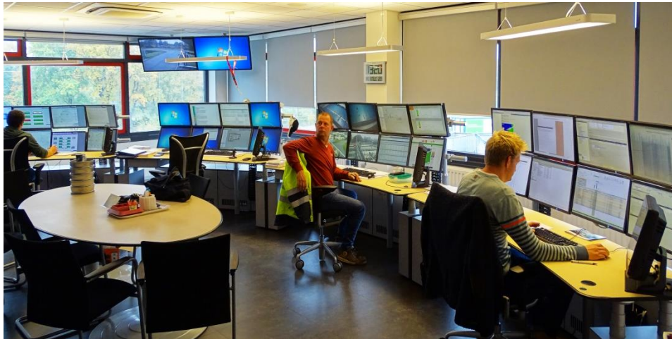
Figure 3 Central control room using TeleControlNet for control of waste water treatment plants
