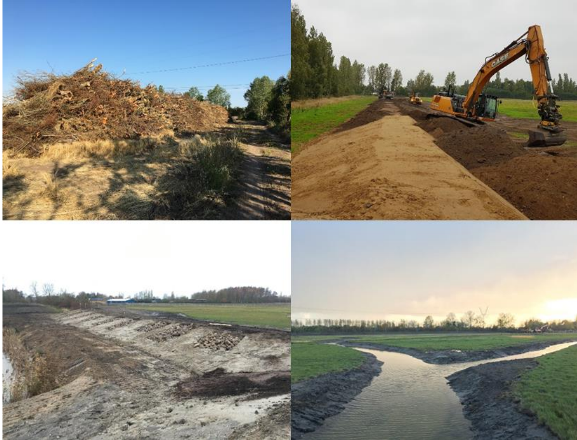
Figure 4-3: Pictures of the specific NbS works. Clockwise from the top left: removal of trees; creation of the new dikes; nature plug ins (the rocky pits in the dike, providing habitats for amphibians); creation of the new watercourse.
