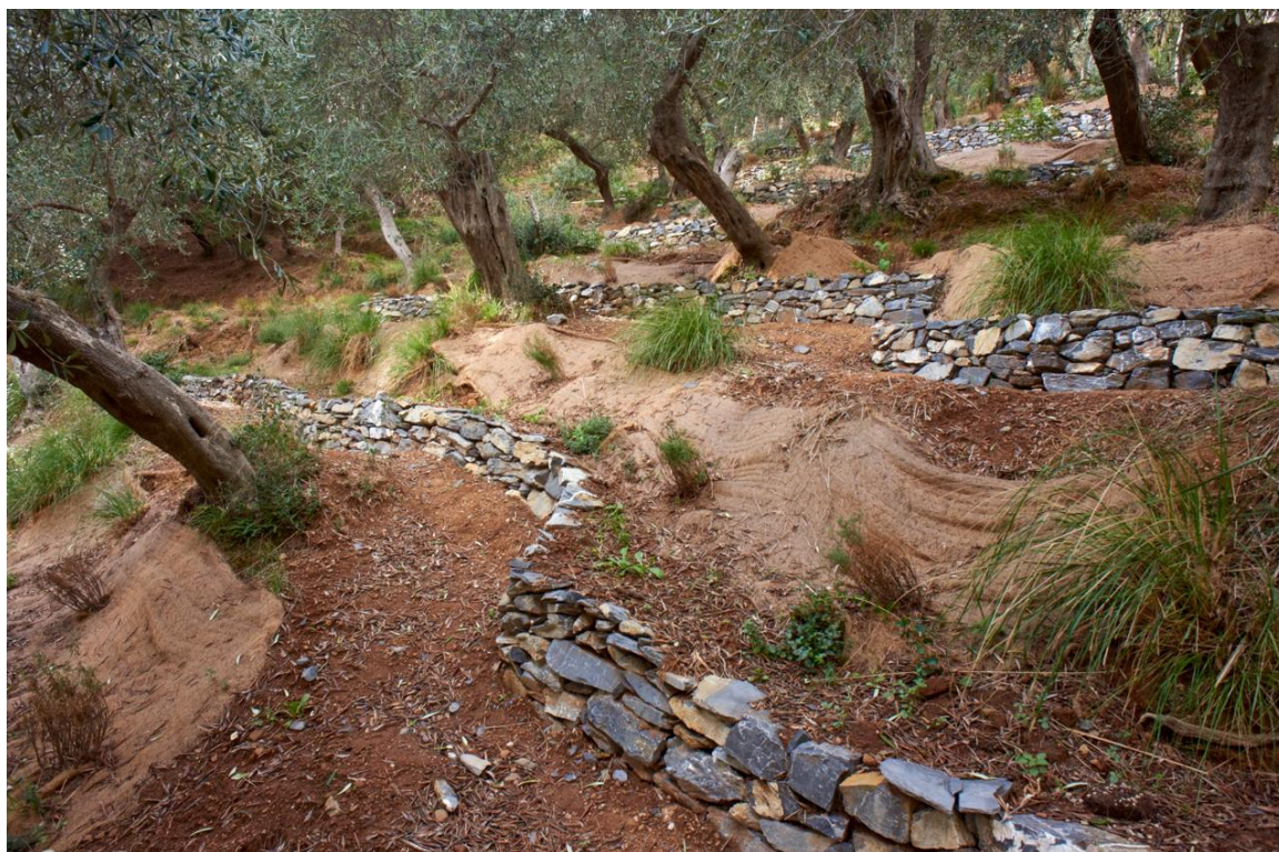
Figure 3-1: Restored dry-stone walls in San Fruttuoso di Camogli. Photo source: GISIG's presentation at the 11 th RECONNECT GA.
