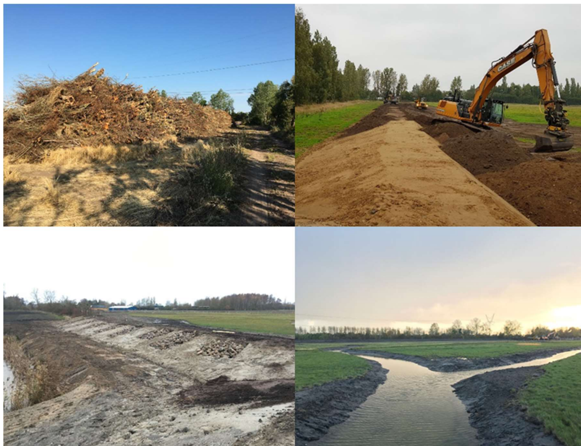
Figure 3-8 Pictures of the specific NbS works. Clockwise from the top left: removal of trees; creation of the new dikes; nature plug ins (the rocky pits in the dike, providing habitats for amphibians); creation of the new watercourse (from D5.4 – Standard for Planning, Design, Implementation, Monitoring, Evaluation of large-scale NbS).
